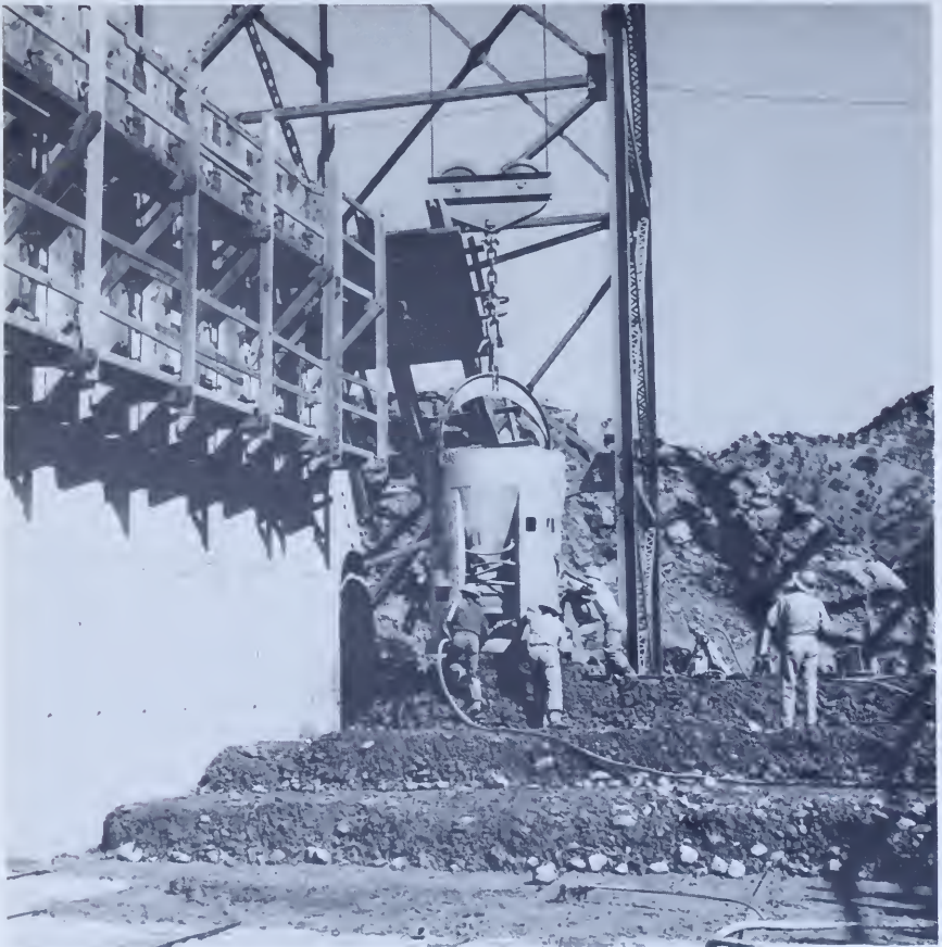
Figure 138.—Step method of placement as used at Monticello Dam, Solano project, California. SO-1038-R2.
